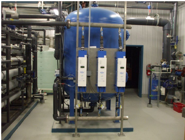
The Original Sand Filter with UV upgrade
