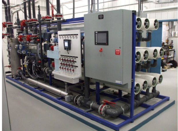
The North RO (new)
