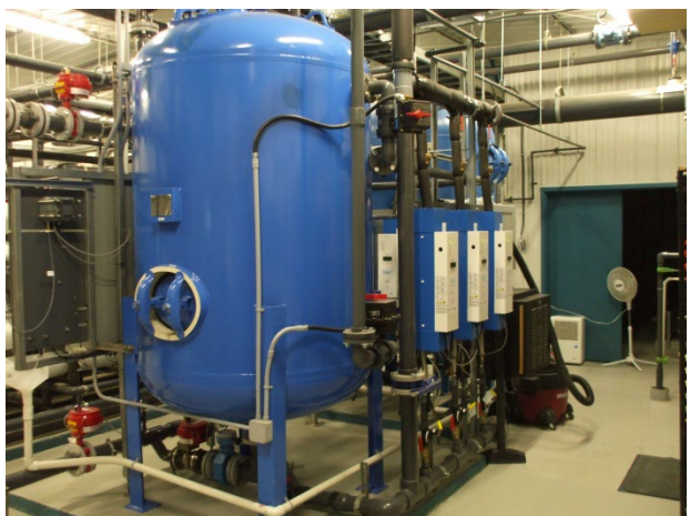
The New Sand Filter with UV
